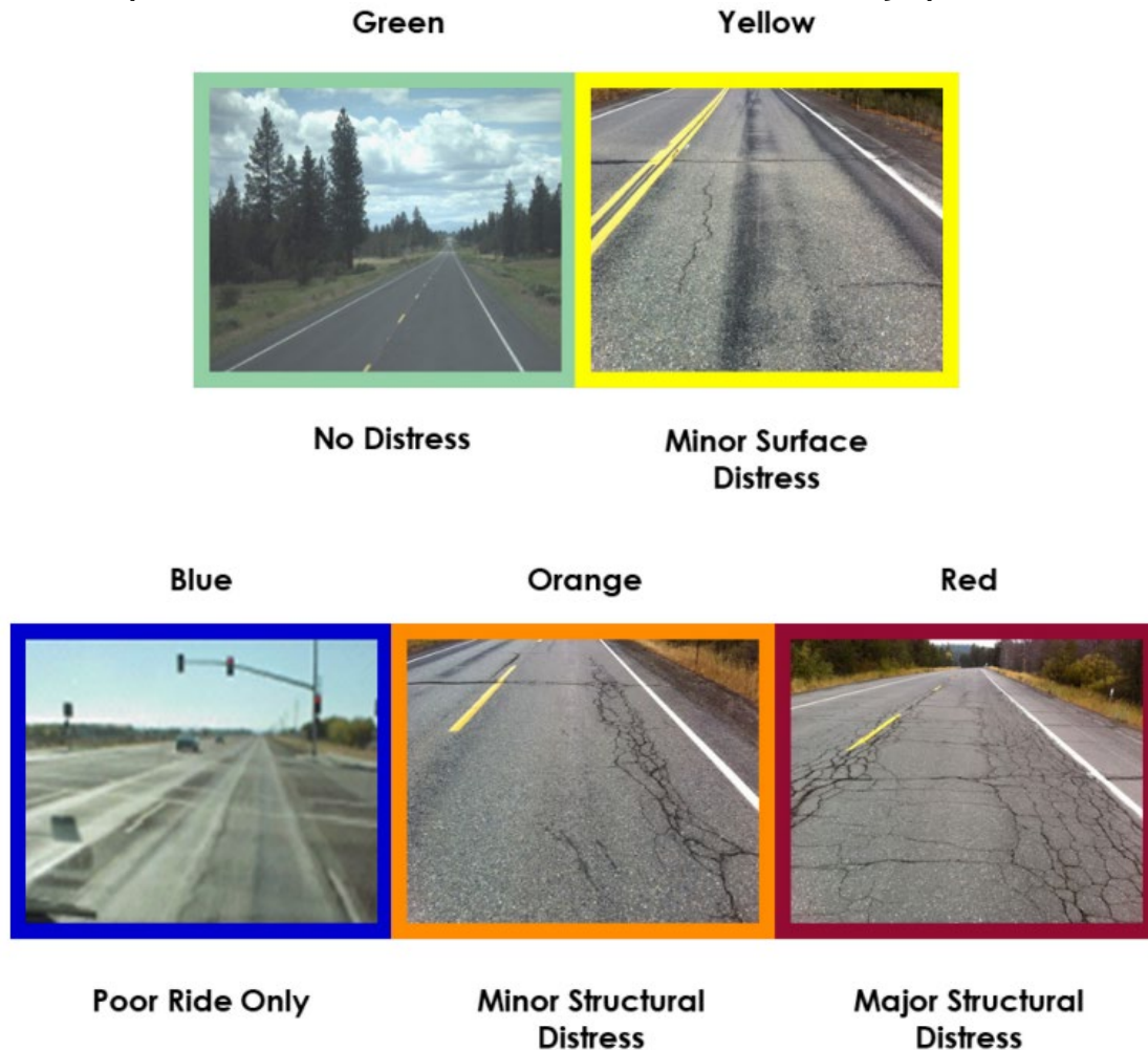
Figure 27: Example of Pavement Conditions based on Caltrans' Rating System
